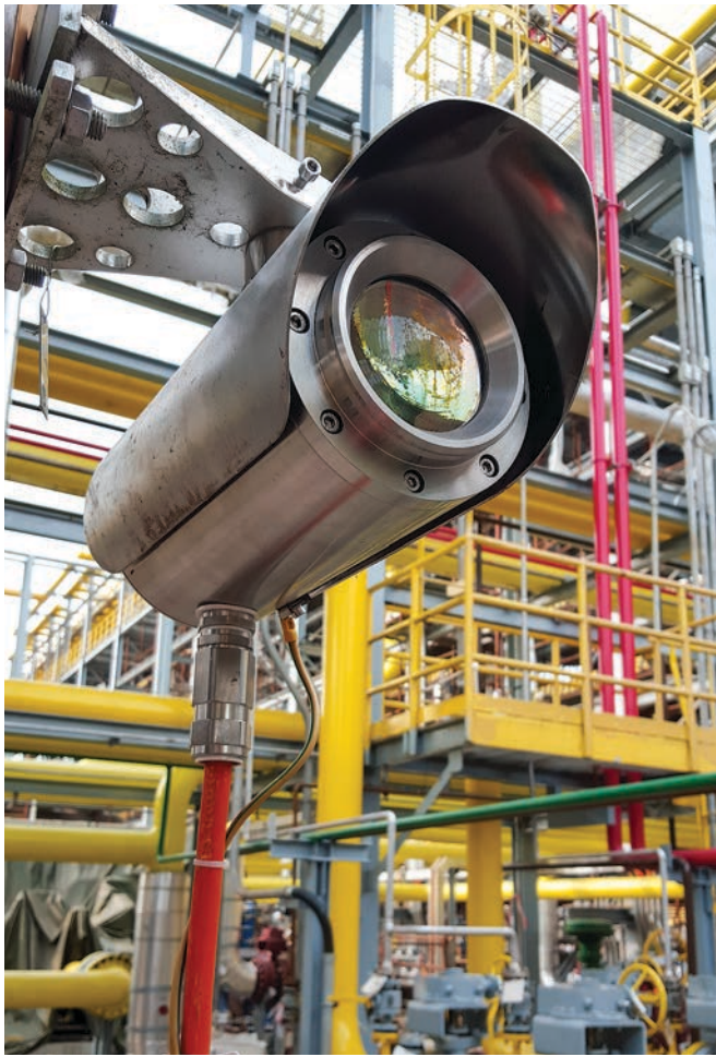
FIG. 2. A gas monitoring system composed of four individual enhanced laser diode spectroscopy (ELDS) open-path HF gas detection sensors was recommended to surround the alkylation unit's processing area.
