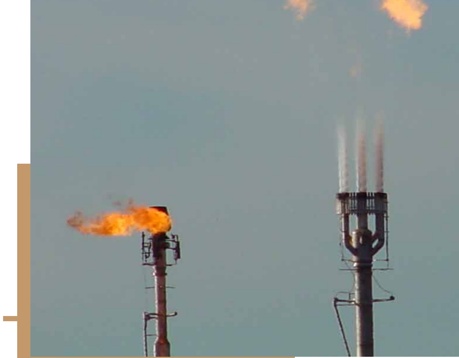
CSF-7-14 Flare Tip Gas plant Alaska
