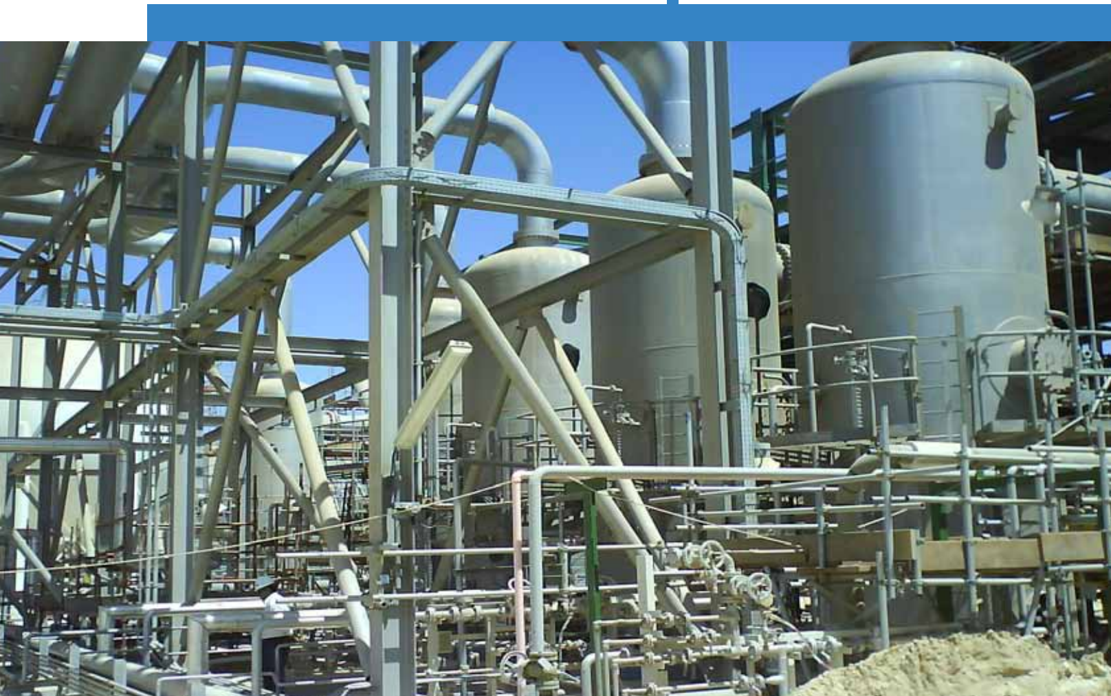
Water Seal Drums Petrochemical plant, Saudi Arabia
