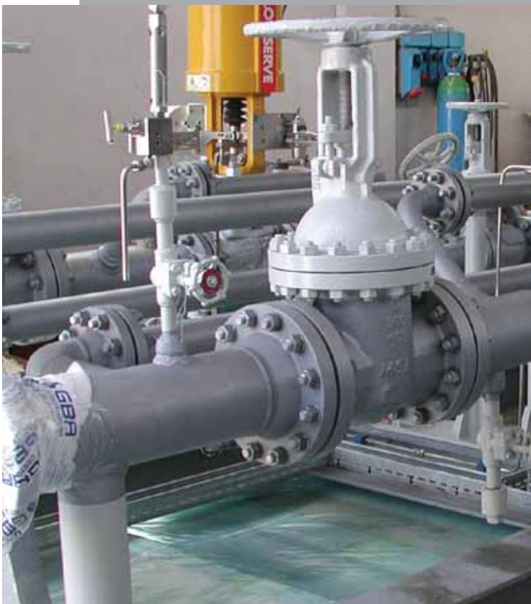
Steam Control Skid Petrochemical plant UAE
