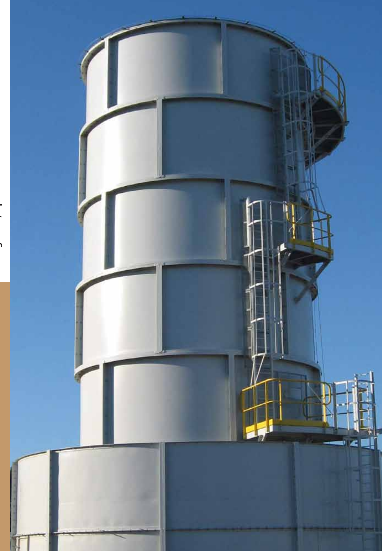
15t/h Enclosed Ground Flare Mugardos, Spain
