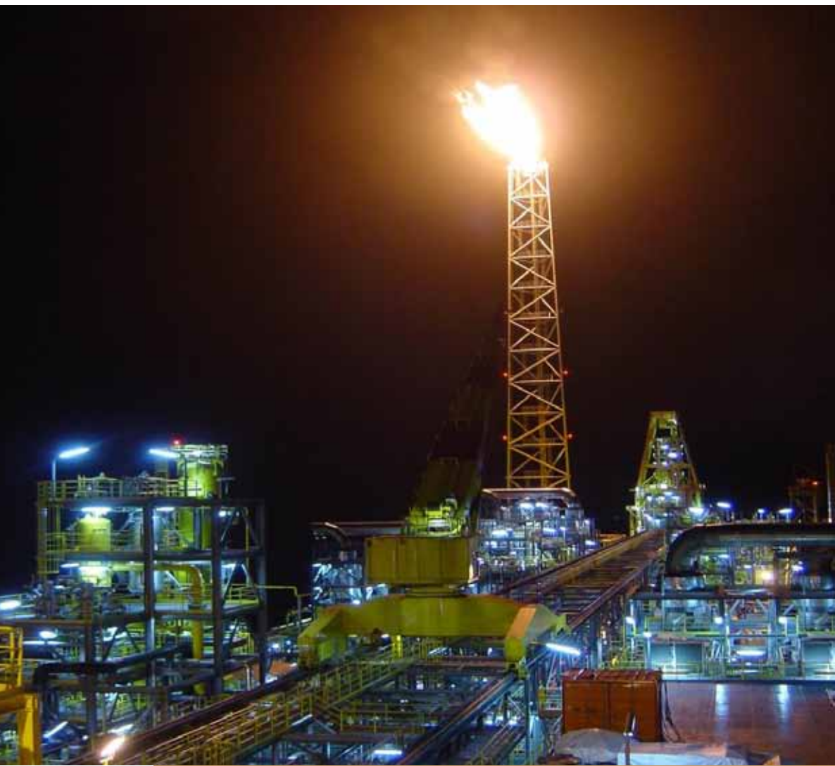
CSF-6-8-HL-14 HP/LP Flare Tip FPSO offshore Nigeria
