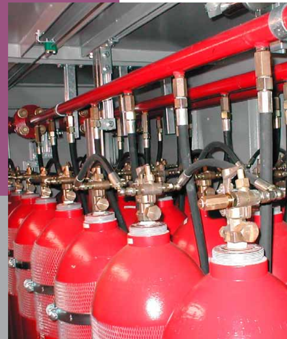
CO 2 Snuffing System Offshore Nigeria
